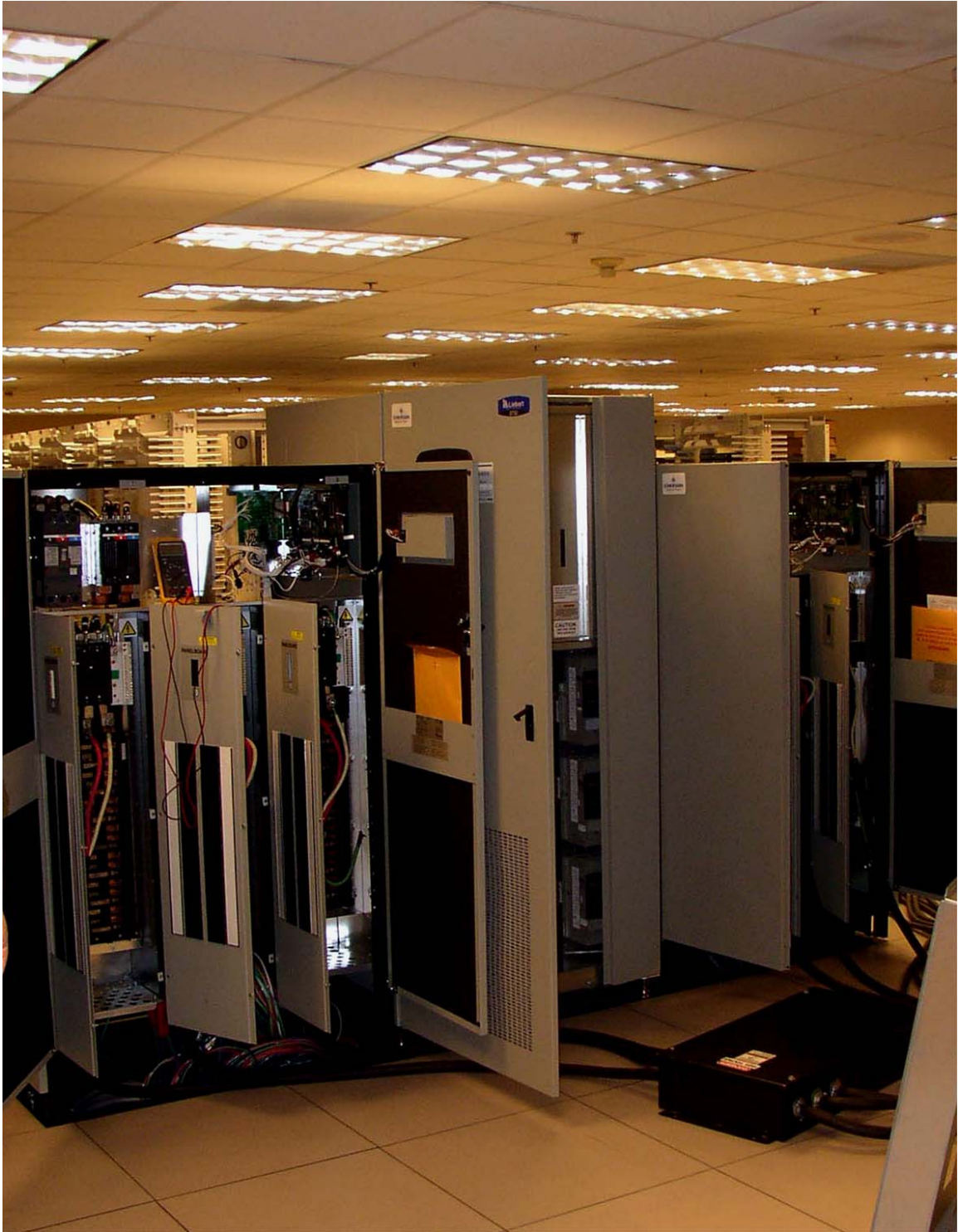
Figure 1 – Typical PDU in a data center with load bank test being run.
